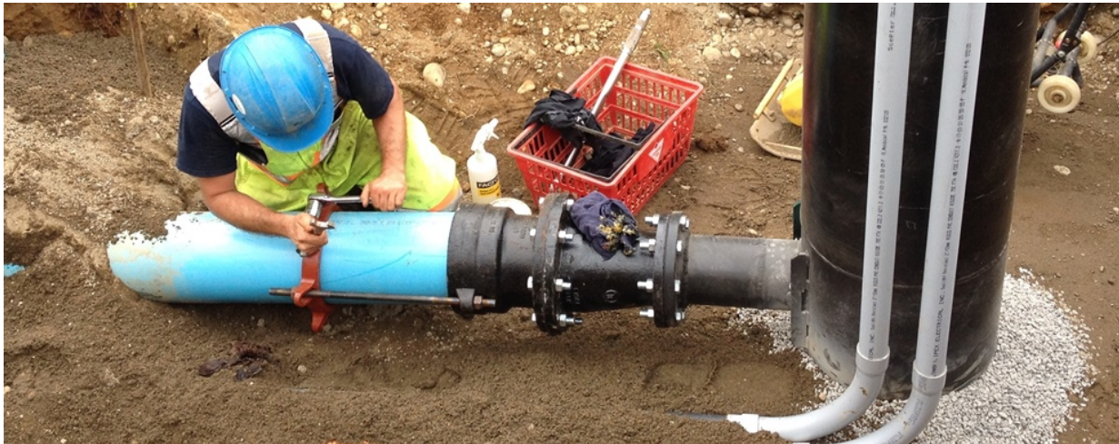
IMAGE | CONNECTING A NEW WATER MAIN SECTION (8 MM BIONAX) TO THE WELL PIT-LESS UNIT
