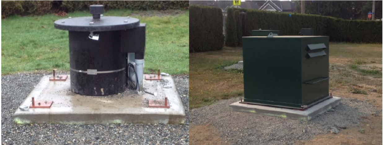
IMAGE | WELLHEAD (LEFT) AND WELL COVER (RIGHT)
