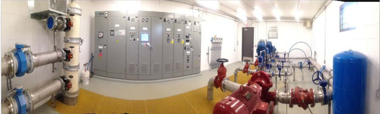
IMAGE | PUMP STATION AT THE RESERVOIR SITE
