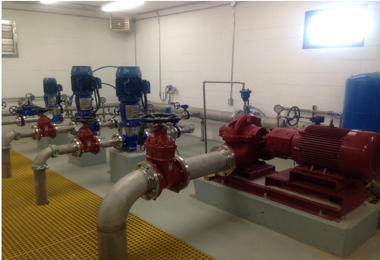
IMAGE | PUMP STATION AT THE RESERVOIR SITE
