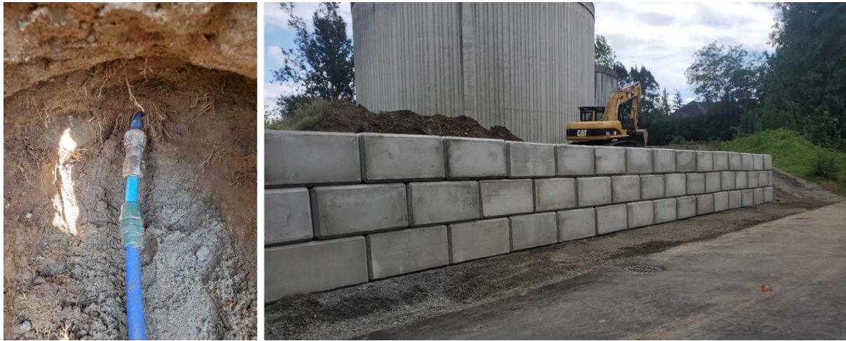
IMAGE | DISTRIBUTION LINE LEAK REPAIR (LEFT) AND NEWLY CONSTRUCTED LOCK RETAINING WALL (RIGHT).
