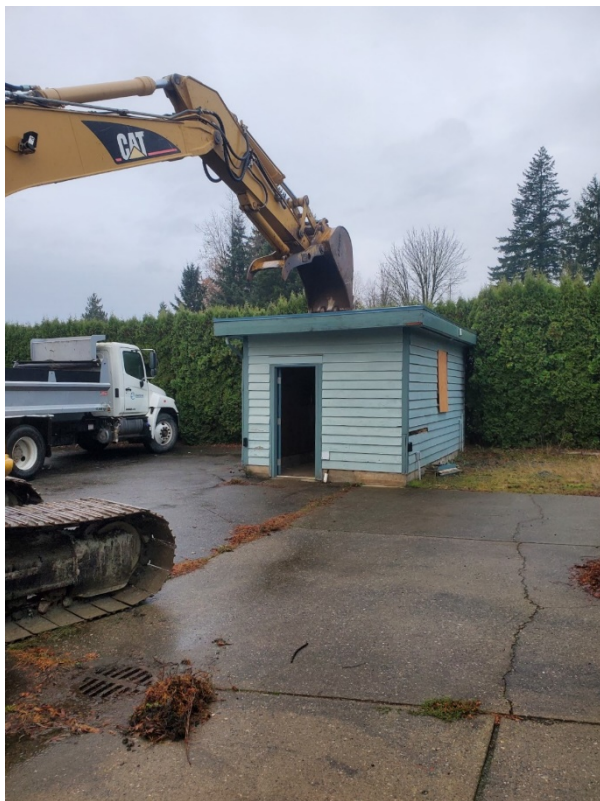
IMAGE | PART OF THE JANZEN YARD & WELL FIELD CLOSURE WAS THE REMOVAL OF THE PUMP HOUSE WHICH HOUSED MONITORING WELL 4-54 (WHICH WAS CWD'S FIRST PRODUCTION WELL)
