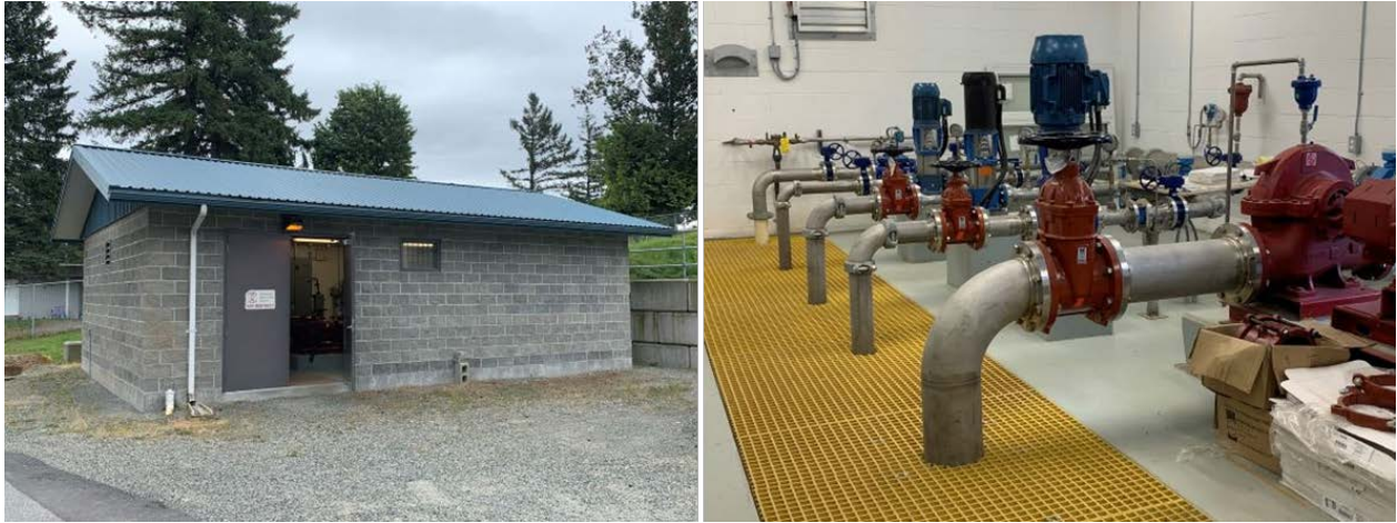
IMAGE | PUMP STATION AT THE RESERVOIR SITE.
