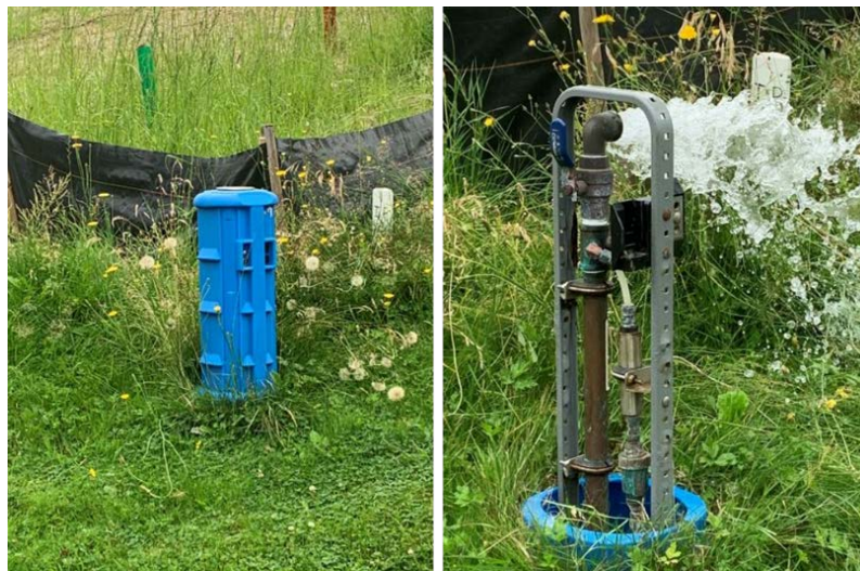
IMAGE | EXAMPLE OF ONE OF THE INSTALLED SAMPLE STATIONS.
